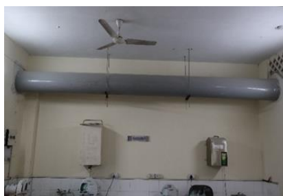
Figure 2b. Adjacent room showing exhaust tube and airflow system
