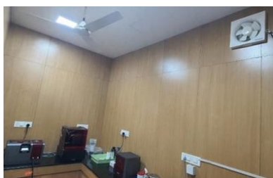
Figure 2a. Ventilated printing room showing exhaust fan
